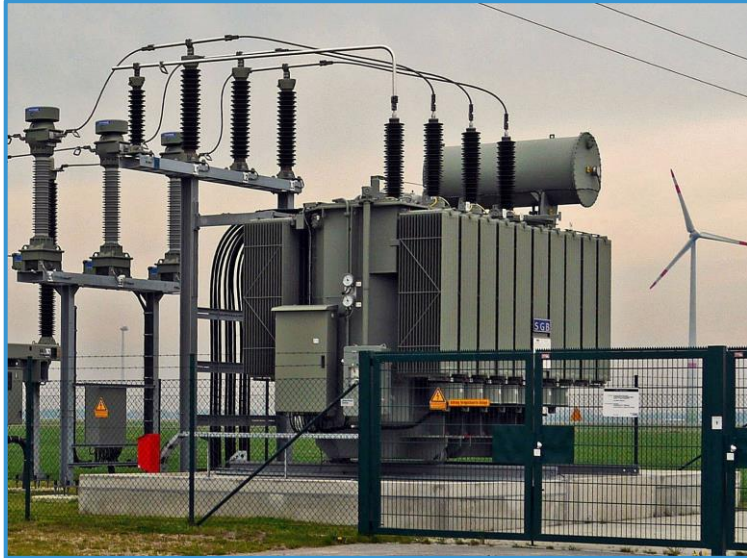
Transformer Condition Assessment
